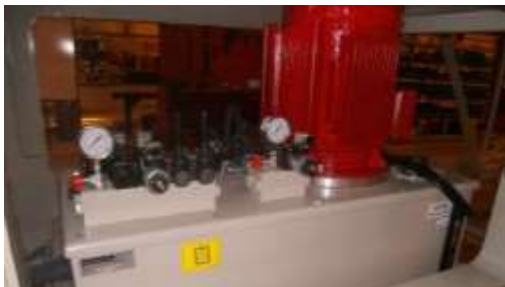
HYDRAULIC POWER PACK
